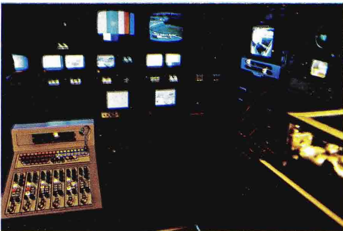
Video Control equipment is housed in the rear compartment. This master engineering center contains all electronic support facilities: joy stick controls for all six color cameras plus video patching, control and monitoring equipment.
