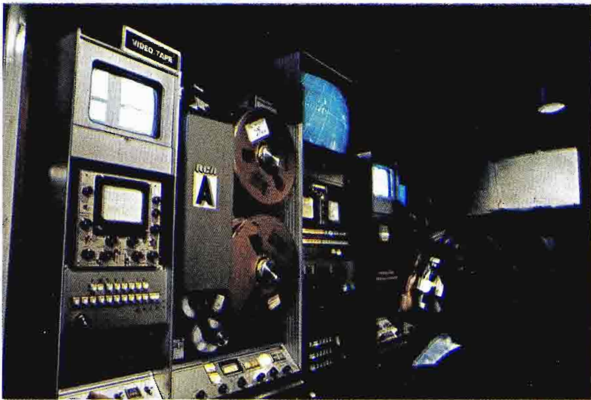
The Video Tape center in the MTS van is located behind the Audio Control and is equipped with two TR-61 VTR's plus tape editing facilities.
