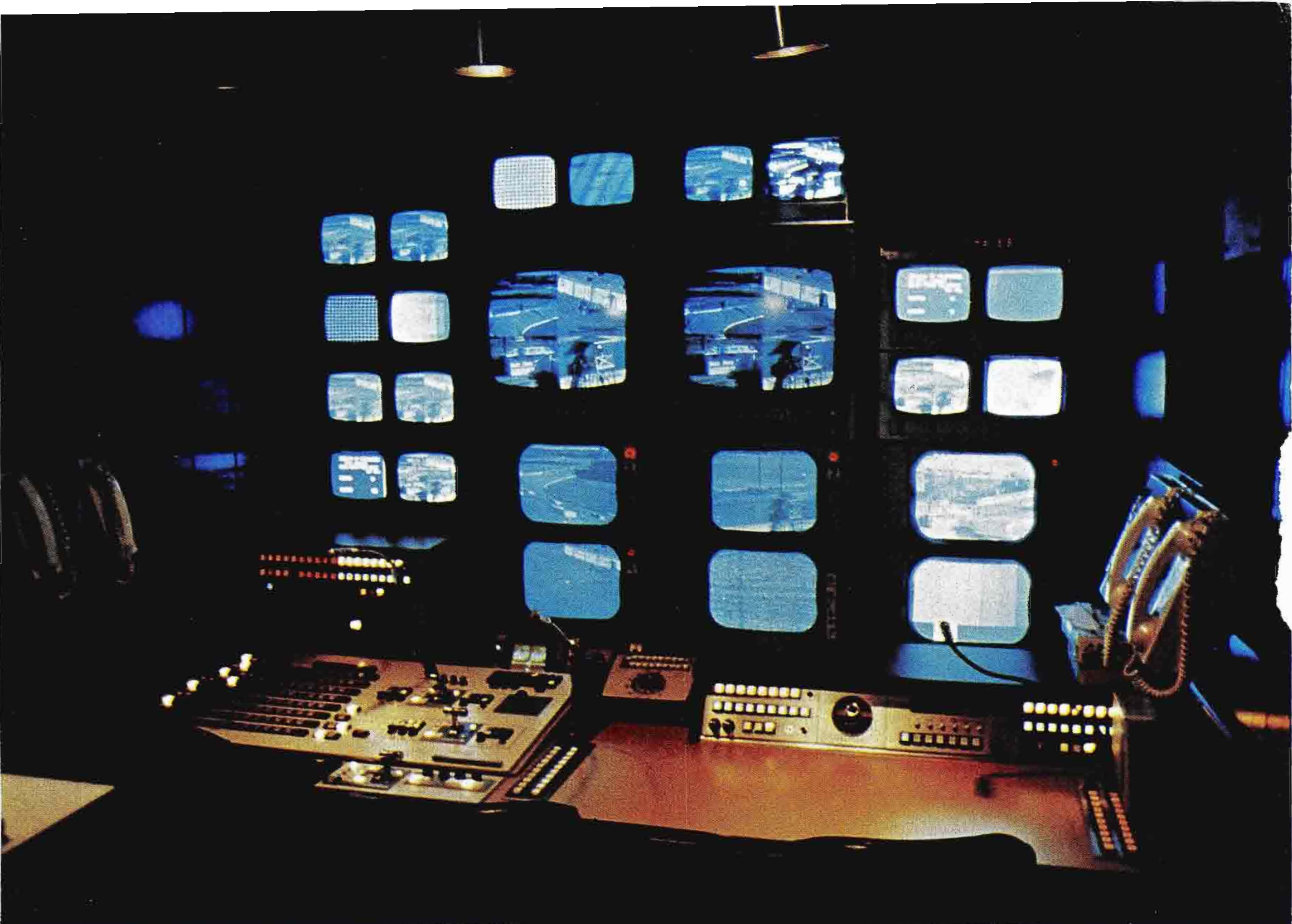
Production Control includes full display of video sources, video switcher with quad split capability; intercom. Space is provided for Technical Director, Director, and Producer/Assistant Director.
