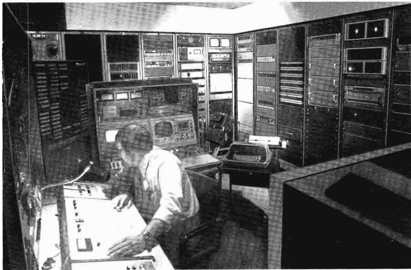
Master Control is unusual in that video and audio equipment racks form two of its walls. The racks back on the engineering shop space, for service accessibility.
