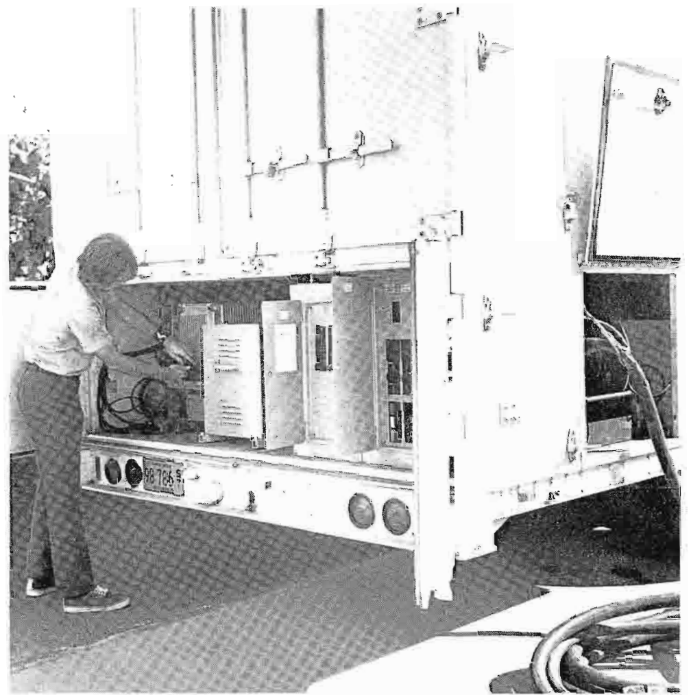
Mounted at the rear of the trailer, behind the video compartment is the power control equipment, including the power input panel; transformers and voltage regulators.
